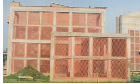
Fig. 6: Red stone 'Jaali wall' used for external facing at TERI Retreat Building at Gurgaon (source: http://www.confoss.com/projects-teri-retreat.html )
